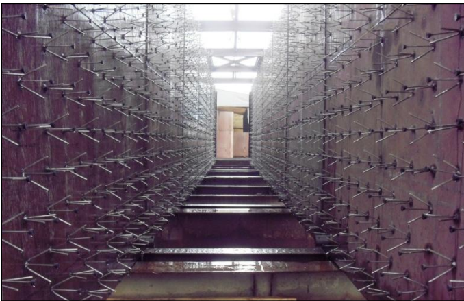
Metallic anchors welded on a convection wall
