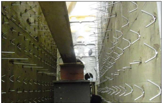
Metallic anchors welded on a convection wall
